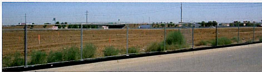
Before installation of the fence, the perimeter sediment barrier was often run over.
