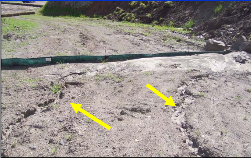
December 2006—two months after installation
