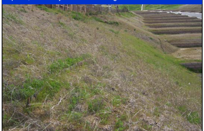
1.5 years after installation—two storm seasons—ProWattle still in place, but barely visible where vegetation has returned
