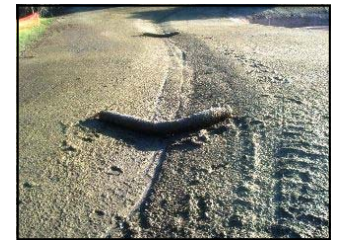
Fiber Rolls were installed first on the site and failed in the first storm
