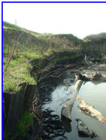
Figure 5: 2 months after install
