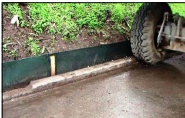
S-Fence™ - protection at base of slope
