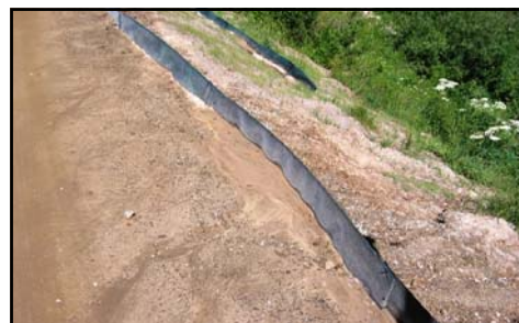
ERTEC spreads flow & captures sediment. It will not let rills and gullies propagate
