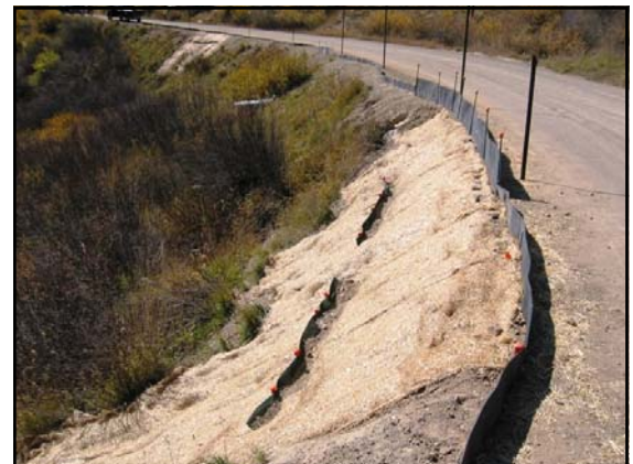
BEFORE: Summer 2010—road is threatened with rilling & head-cutting
